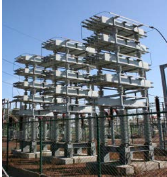
Figure 1- Capacitors being used to correct the power factor in industries
